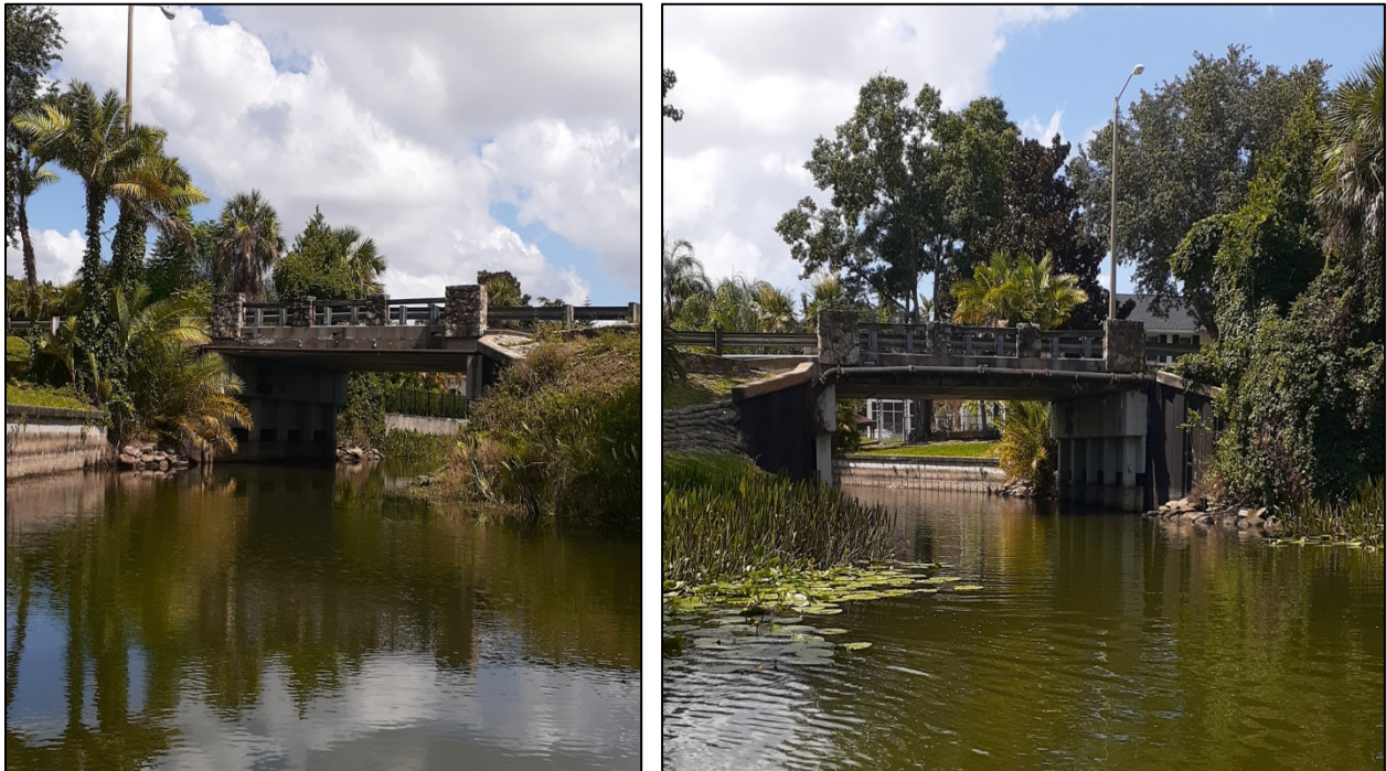
Photo 4-1: Gatlin Canal (5/4/2021, 5/5/2021) - The canal had little vegetation near the bridge and no vegetation in most of the canal
