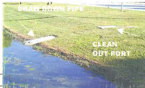
The South Filtration System
