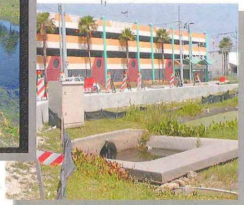
Concrete Lined Sediment sump
