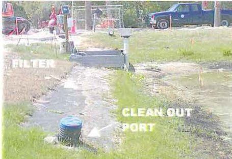
The North Filtration System
